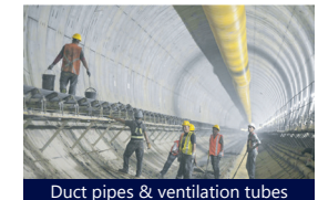
Duct pipes & ventilation tubes
